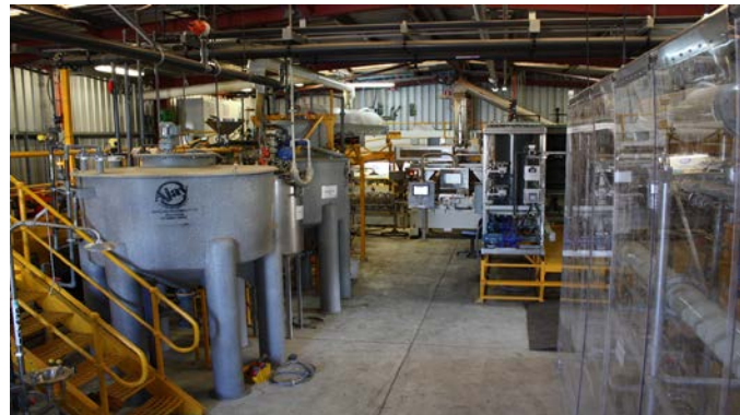
Australia, @ The Ehtec Lignocellulosic Bioethanol Pilot Plant in Muswellbrook
